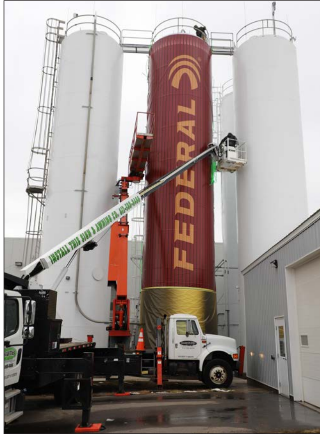
A contracted crew places a sleeve over a silo at the Federal ammunition plant in Anoka on Oct. 23 to make it look like a shotgun shell. The silos contain plastic resin, which comes to the plant by rail and is pumped into the silos.
