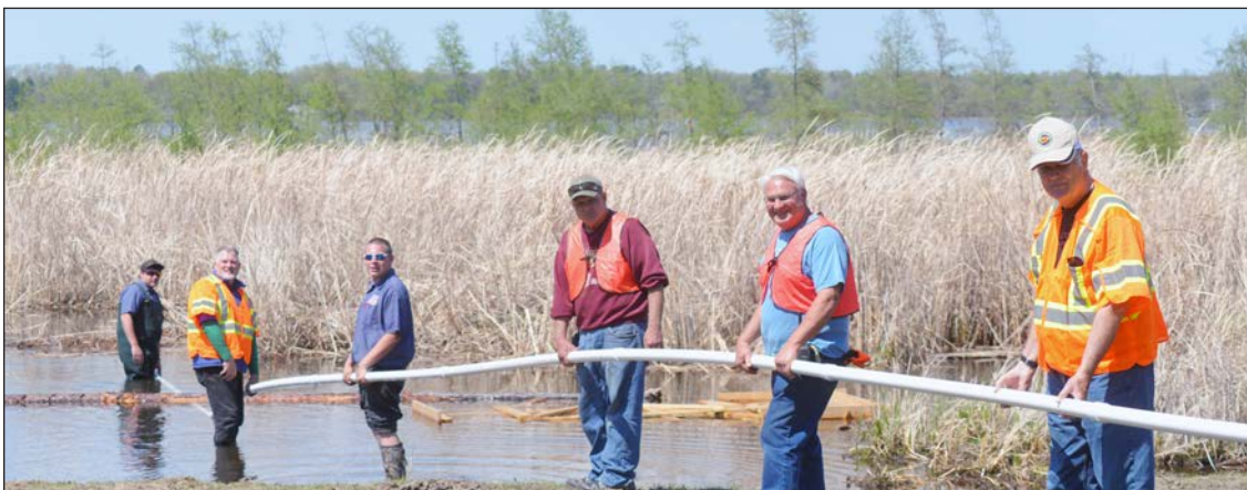
Volunteers try to push a 200 foot section of PVC pipe under the bog. A rope in the pipe then could be used to pull a cable under the bog and then dragged back through, cutting the bog in half.
